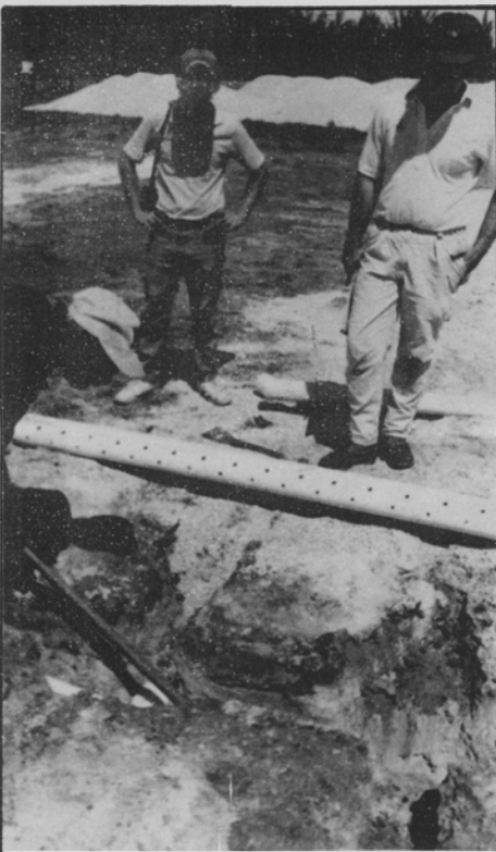
Local Golf Course Maintenance crews diligently work on construction of the IFAS Research Green at Fort Lauderdale this past month.
