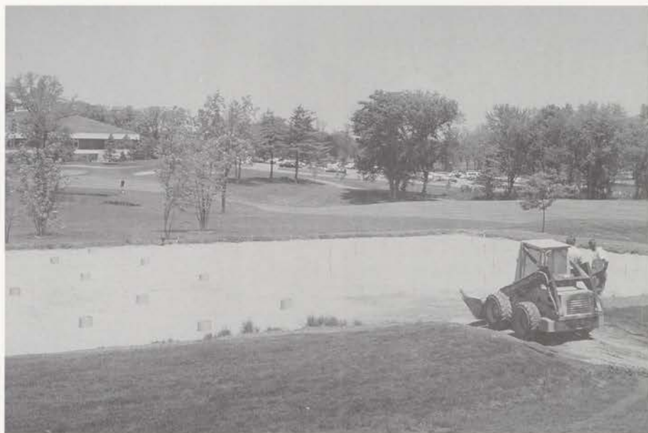
Cantigny Green construction in June 1994 prior to addition of the root-zone mixes.
